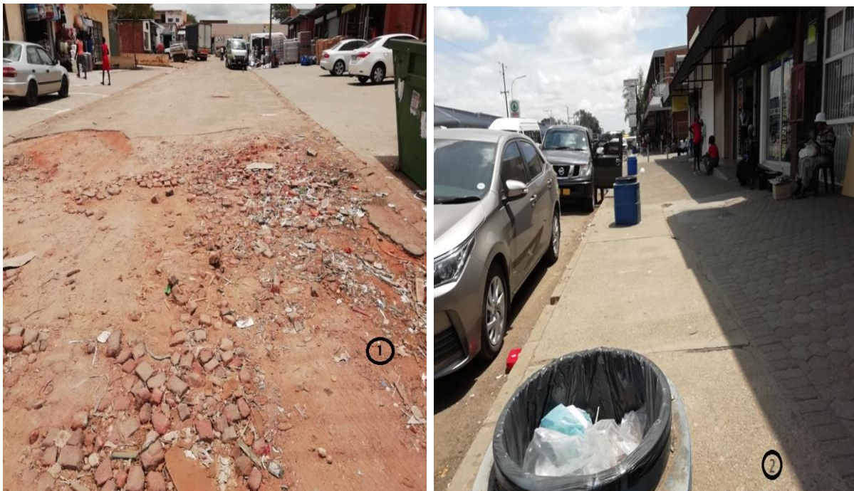
Photograph 6-7: A street with potholes in Musina Town
