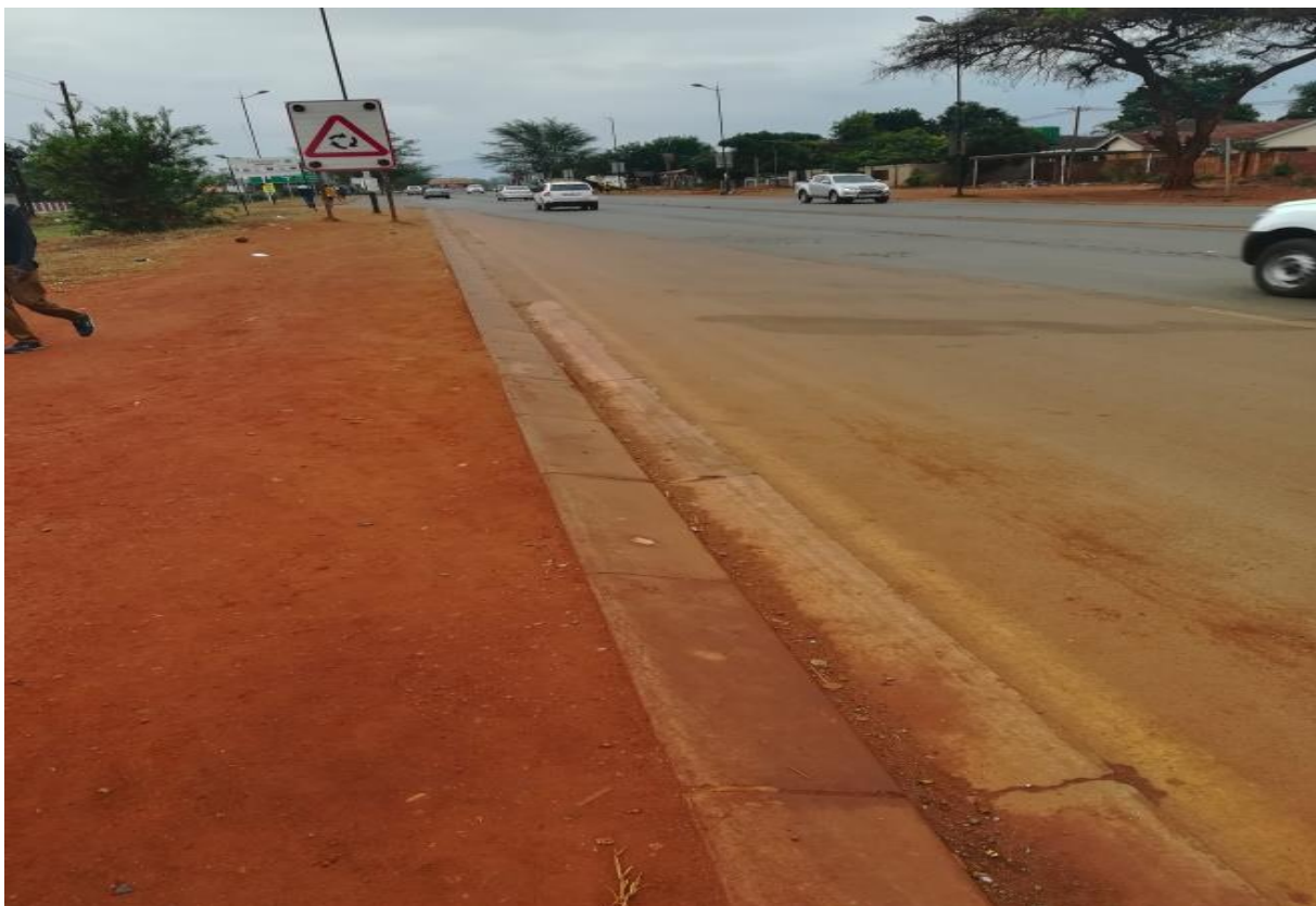
Photograph 5-4: An unpaved sidewalk in Thohoyandou Town Source: Research survey (2019)
