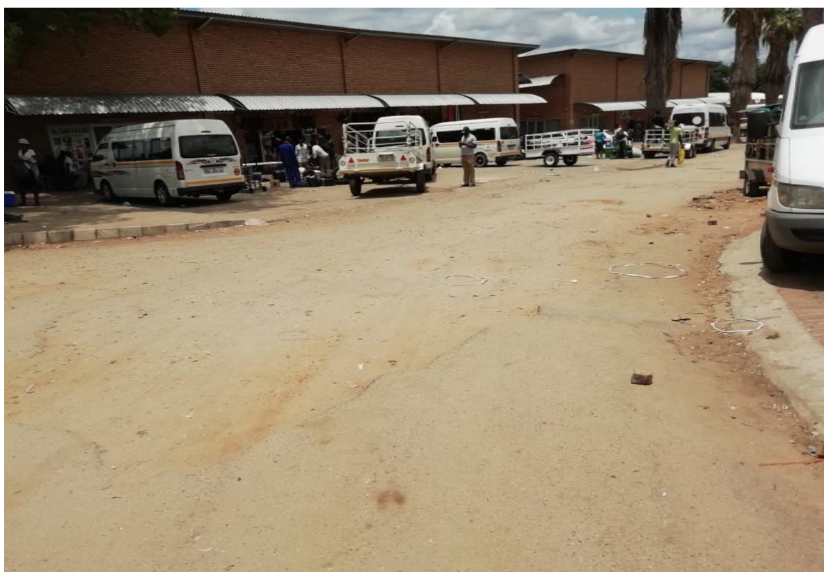
Photograph 7-3: Example of street spaces that require resurfacing in Musina Town Source: Research survey (2019)
