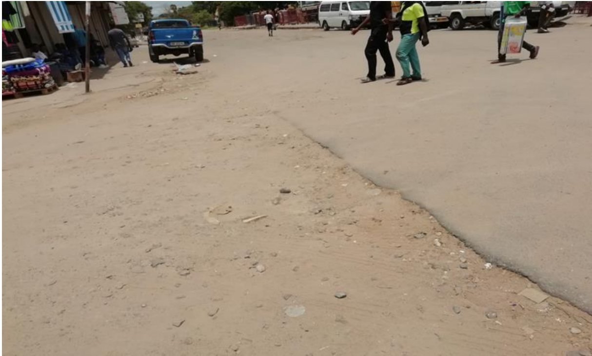
Photograph 5-2: Crosswalk with no clear markings in Musina Town Source: Research survey (2019).
