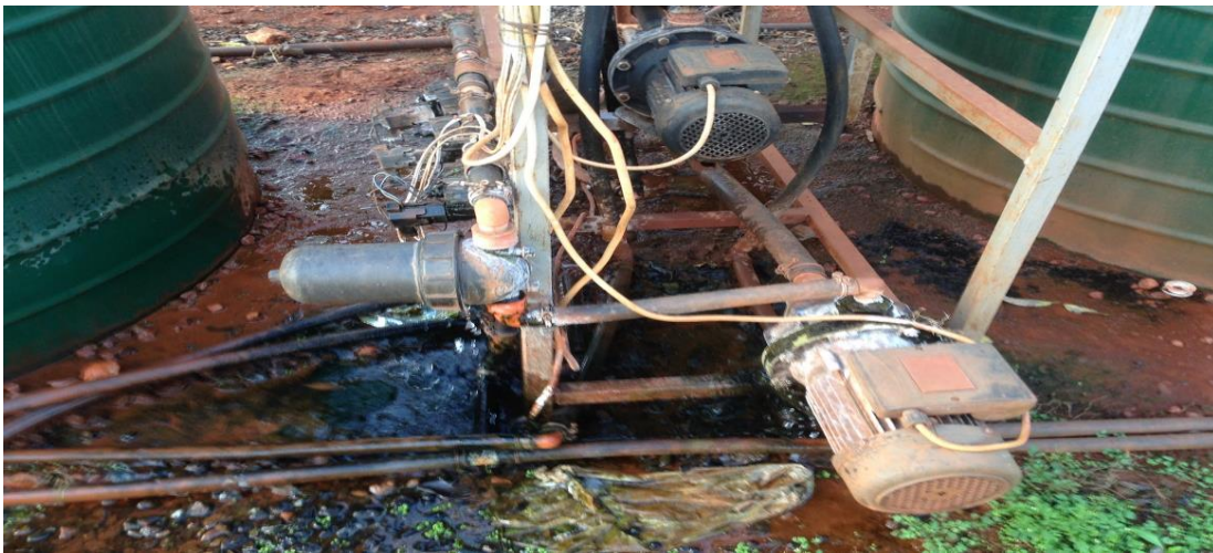
Figure 4.16: Water leakage at the reserve storage located at School of Agriculture
