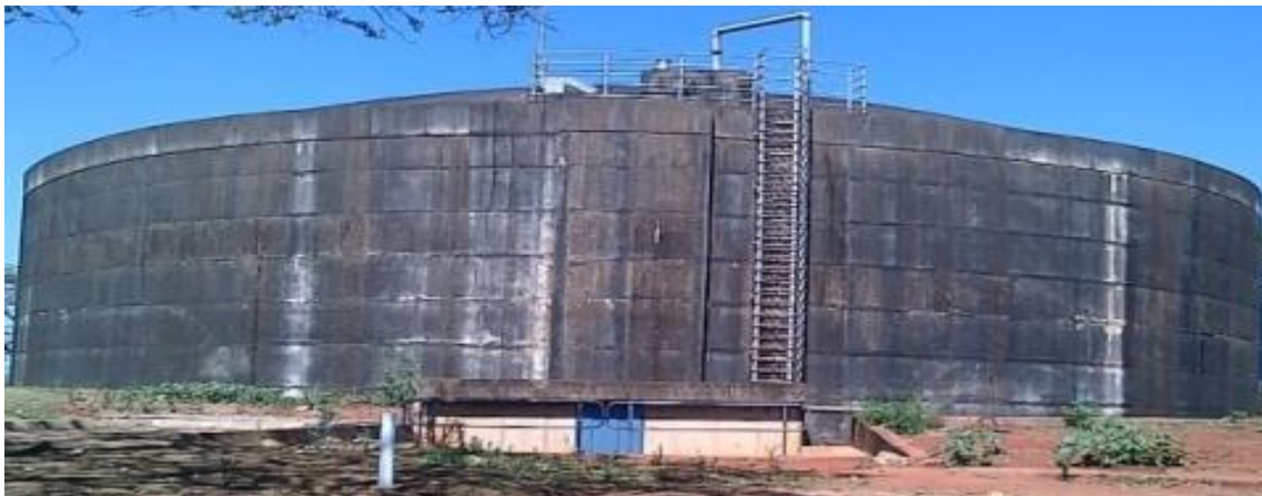
Figure 4.2: Storage reservoir storing water from Phiphidi water treatment
