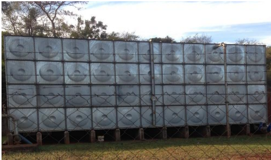
Figure 4.3: Abeco steel tank carrying water from the municipal reservoir
