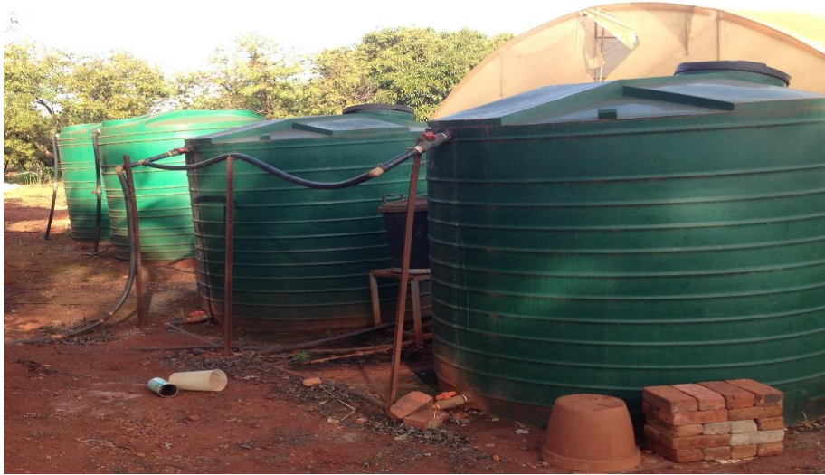
Figure 4.4: Reserve storage tanks located at the School of Agriculture
